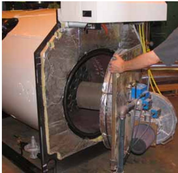
Figure B6-4. Burner maintenance
