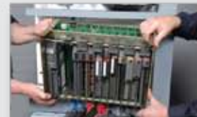
Remove the 1771 chassis from the control cabinet.
