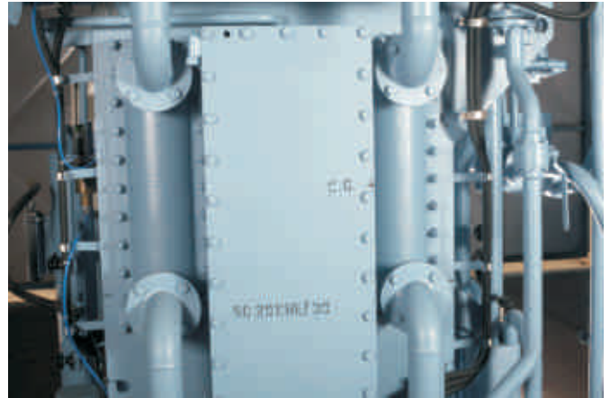
Side-by-side Evaporator and Absorber
