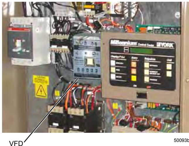
FIGURE 45 - TYPICAL VFD LOCATION
