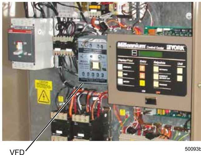
FIGURE 45 - TYPICAL VFD LOCATION
